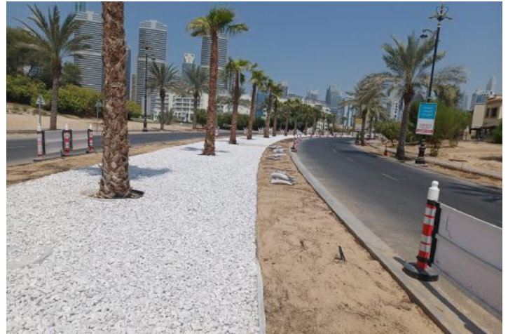
Phase 2 landscaping works in progress at Gate 2. Plantation of ground cover will commence in mid September.
