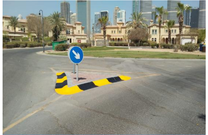
Painting of speed humps and pedestrian crossings will take place starting mid-September (After)
