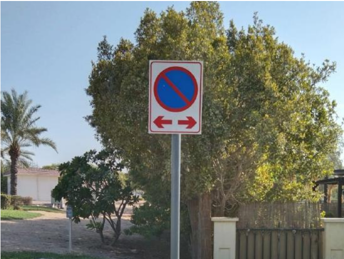
Installation of No Parking signage at Cluster 22 & 24 junction to ensure free flow of vehicular traffic
