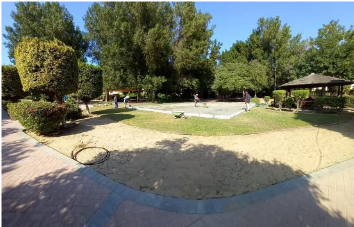
Teqball flooring installation works in progress at Al Rawdha Park near Clusters 43 and 45.
