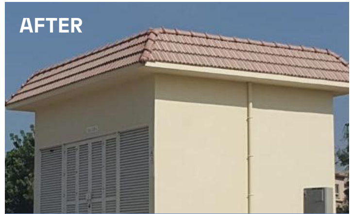
All 38 substations are currently under repair with plaster repair works and a fresh coat of paint being applied.
