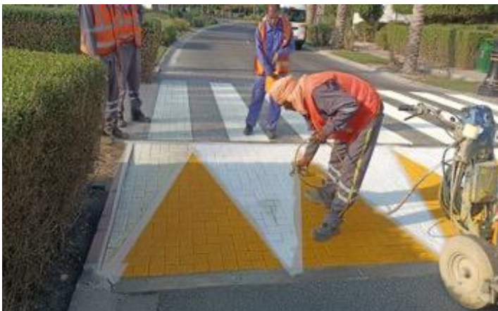
Pedestrian crossings needed a paint refresher.
